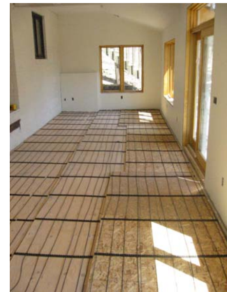
During construction: the in-floor heating being laid in the new family room.
