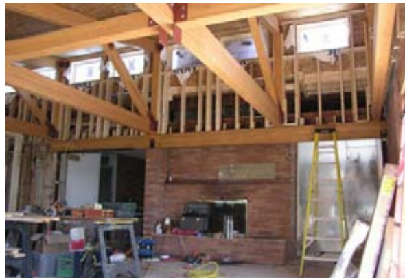
Structural insulated panels (SIP) on top of trusses, framing of clerestory wall
